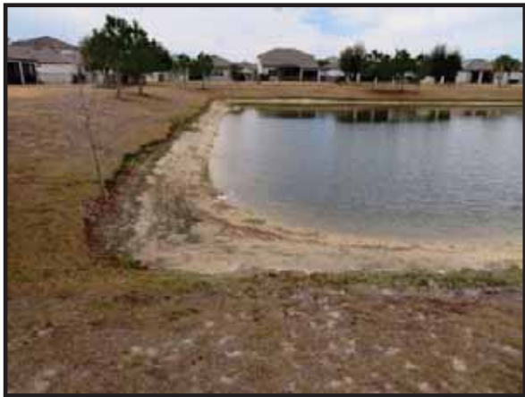
Figure 3 - Pond 28 Shoreline Erosion
